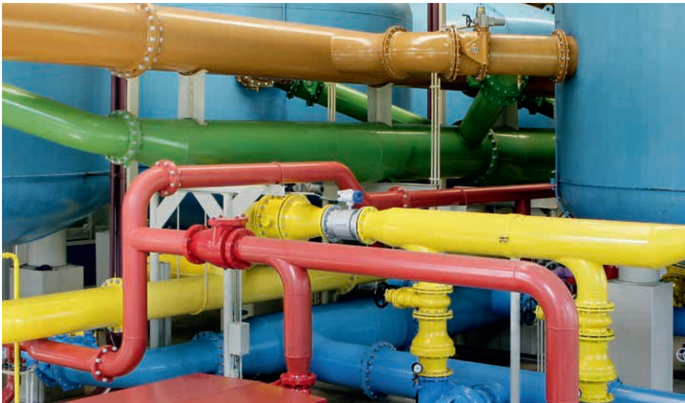
OPTIFLUX 4300 in the filtration system in the Haltern waterworks, Germany
