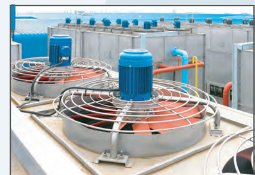
Fan and water pump
